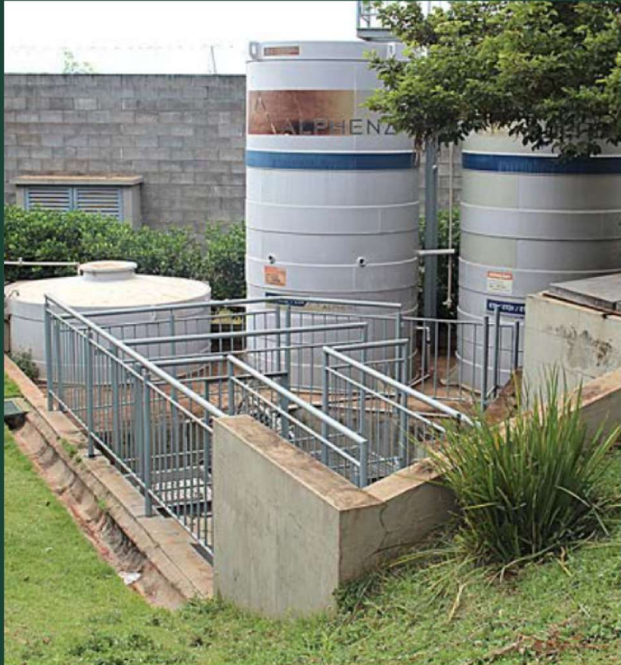
Effluent treatment station (ETE) at BYD's plant in Campinas (SP).
