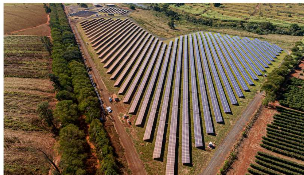
BYD Brazil's R&D photovoltaic plant
