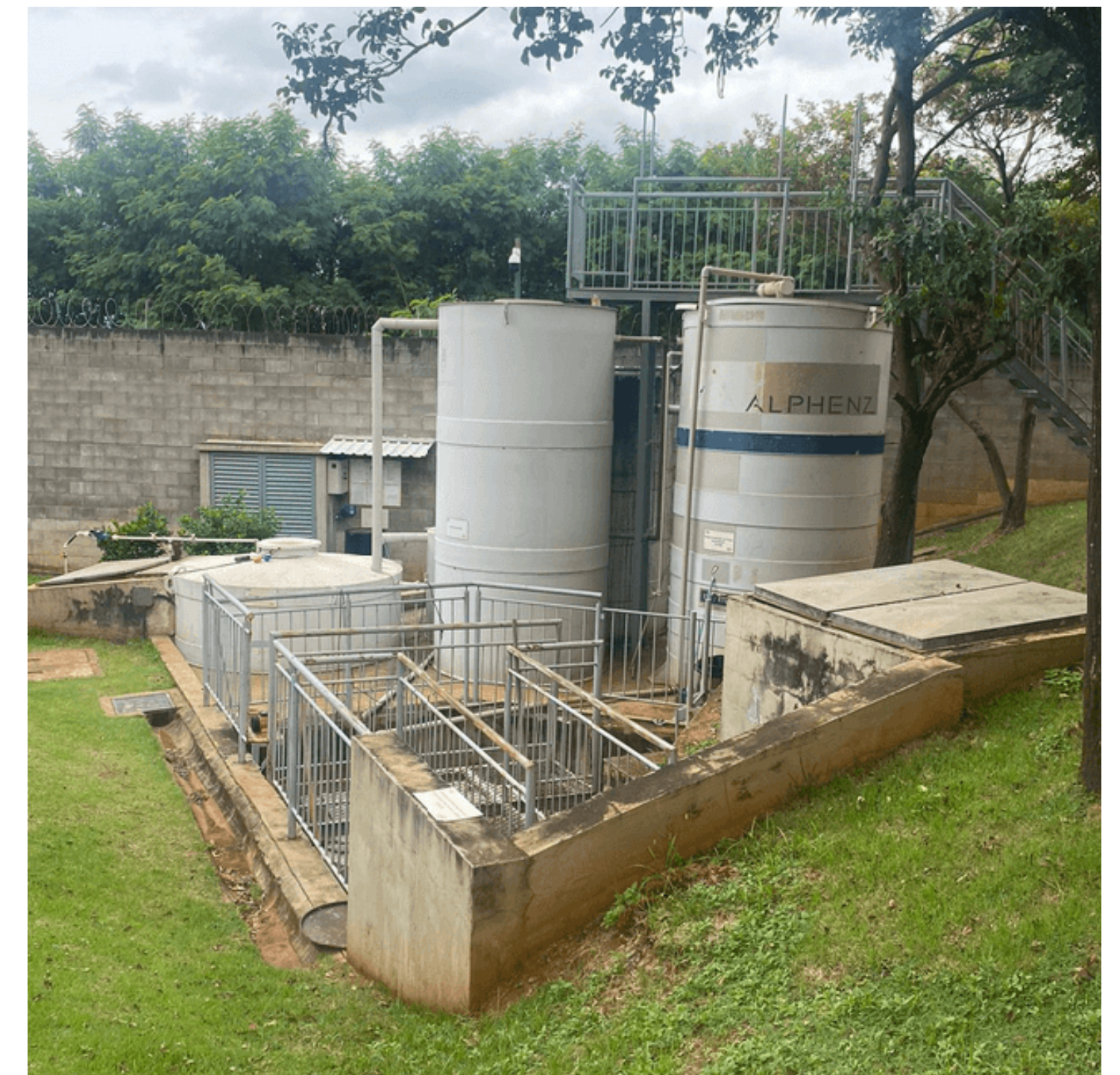
Effluent Treatment Plant (ETP) at the BYD factory in Campinas, São Paulo
