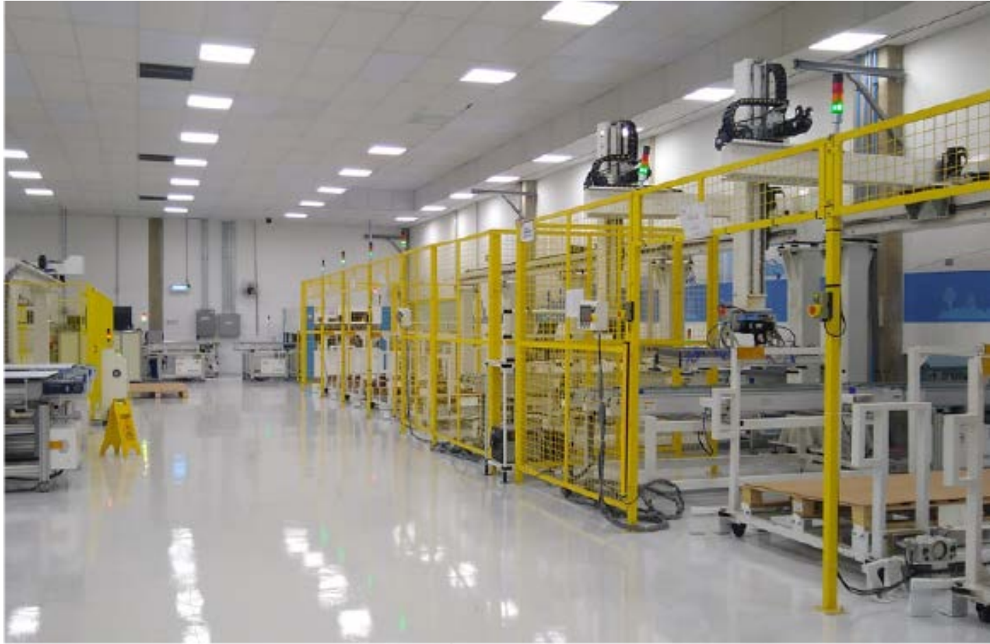
LED lamps installed at the BYD Energy factory in Campinas, São Paulo
