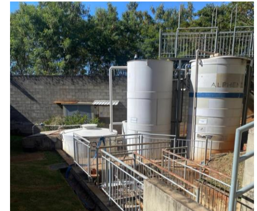
Effluent Treatment Plant (ETE) at BYD Brazil's factories in Campinas (SP)
